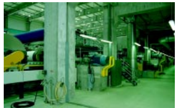
The system included 47 motors ranging in power from 37 kW to 1690 kW.
