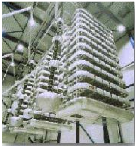
HVDC Thyristor Valves
