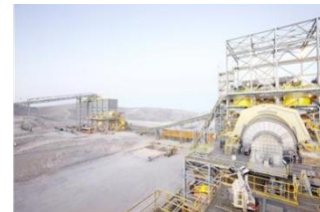
Gearless conveyor drive system for world's largest underground copper mine in Chile
