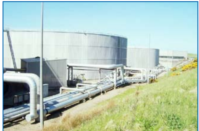
Scottish & Southern Energy, Peterhead power station
