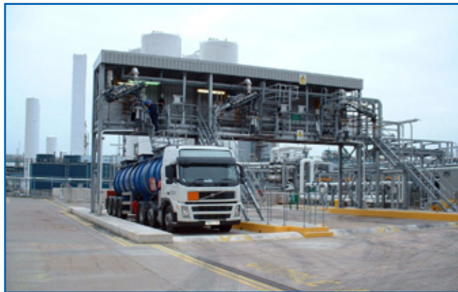
The fully operational Hypochlorite Storage and Loading Facility
