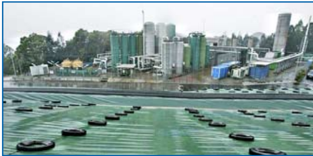
Existing landfill gas plant in North East New Territories (NENT), Hong Kong
