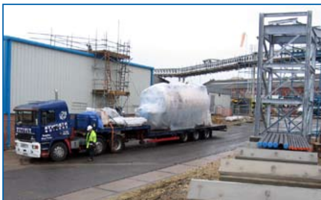
Pipebridges and boiler house at Rohm & Haas
