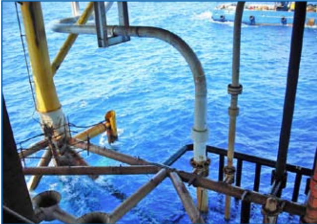
Gas pipes in the North Sea
