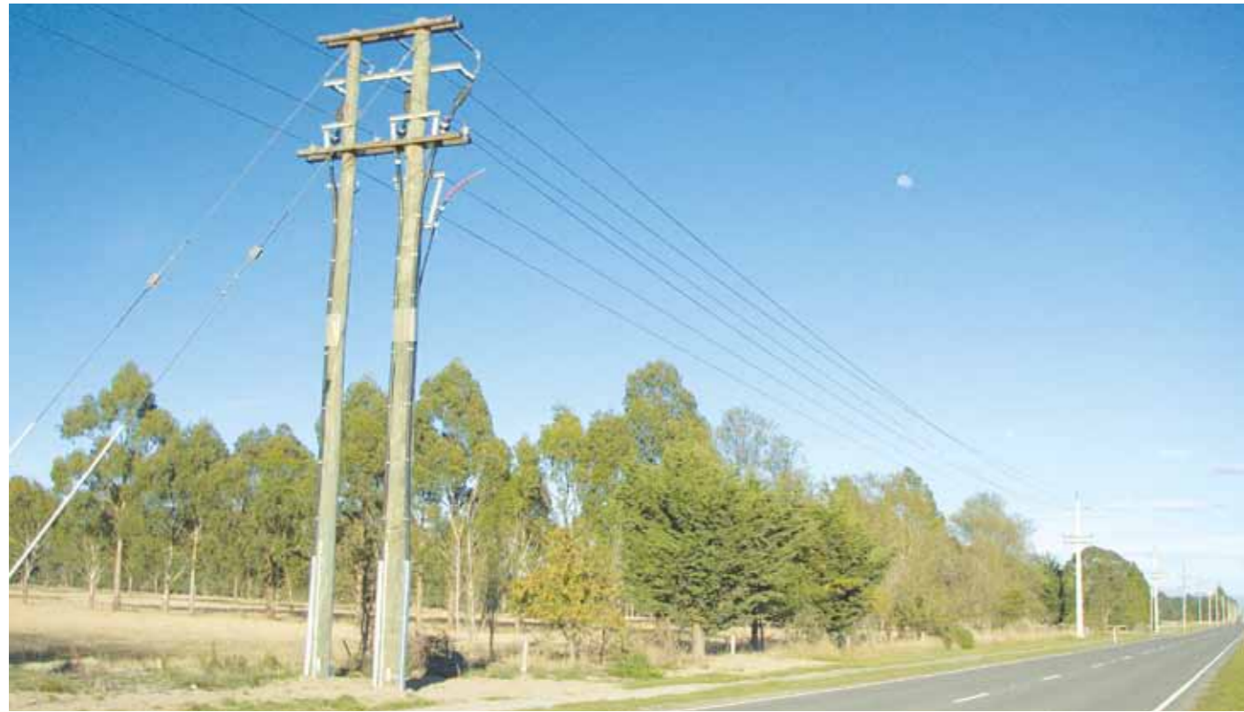
The newly upgraded 66 kV Swannanoa line meeting the energy demands of agricultural irrigation in North Canterbury
