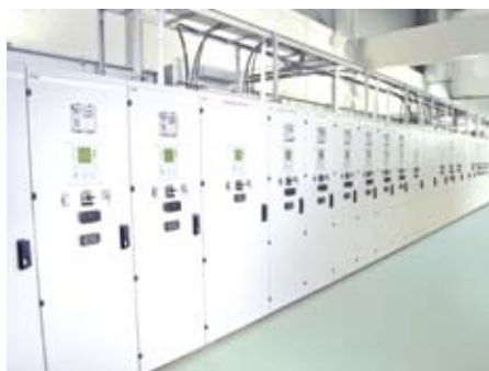
Powering a city's distribution network (10)
