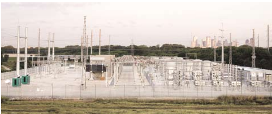
Installed and commissioned by ABB, the SVC (FACTS) installation at the Parkdale substation, in the Dallas/Fort Worth area of Texas is the world's largest cluster of SVC technology.
