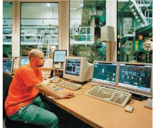
Three ABB quality control systems perform online quality control on PM 6, 7, 8 and the flash dryer.
